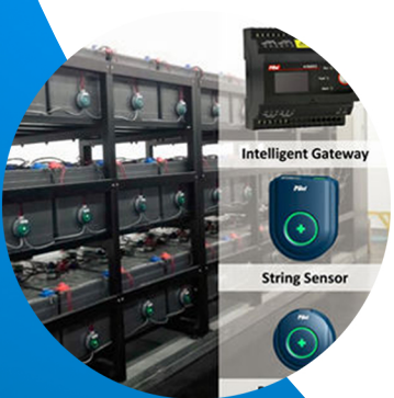
Battery Monitoring Systems
