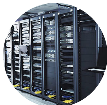
Infrastructured Data Center
